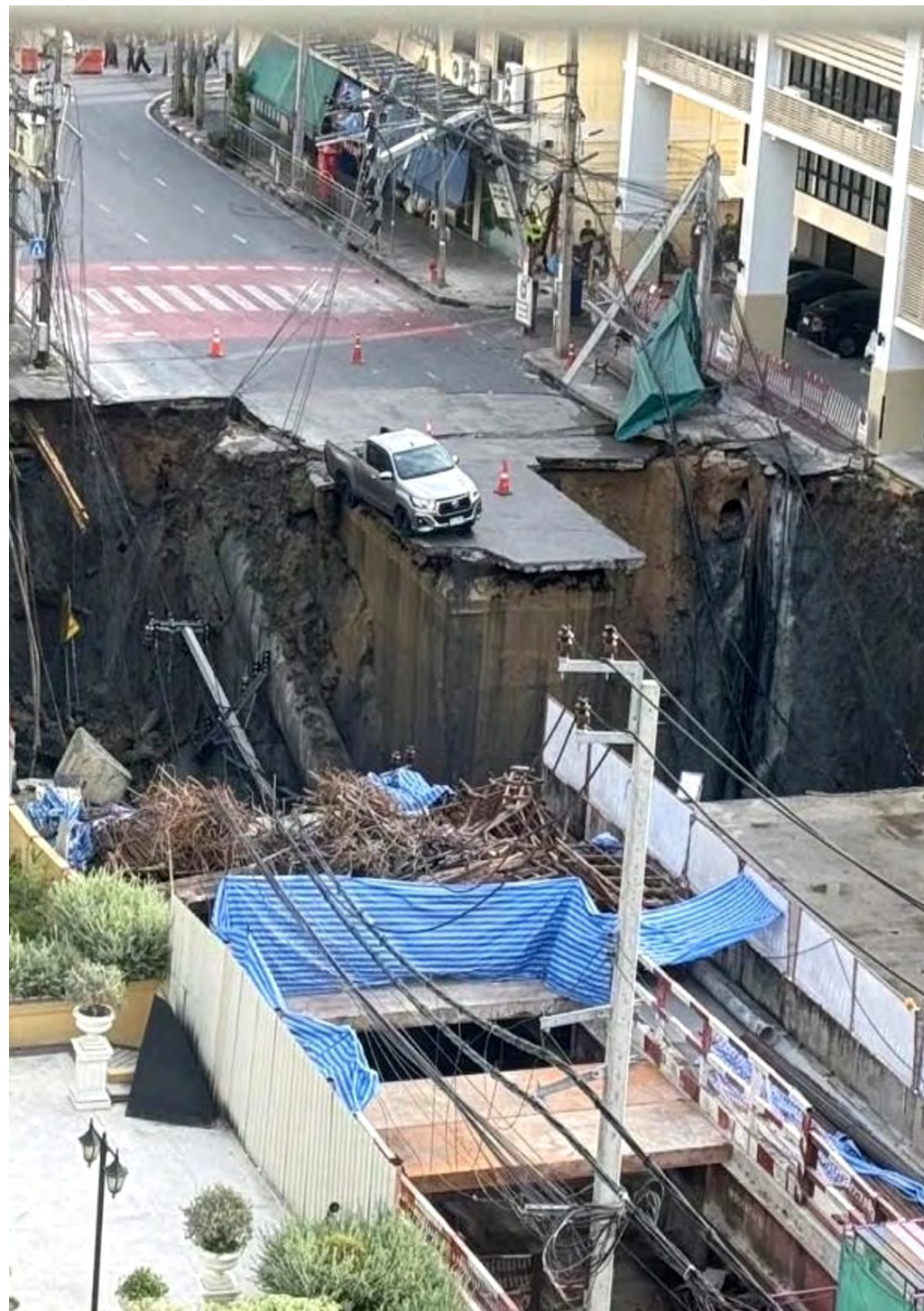
Figure 1. Road subsidence between Vajira Hospital and Samsen Police Station, Bangkok, Thailand on September 24, 2025. Photo: Creative Commons/Wikimedia.
