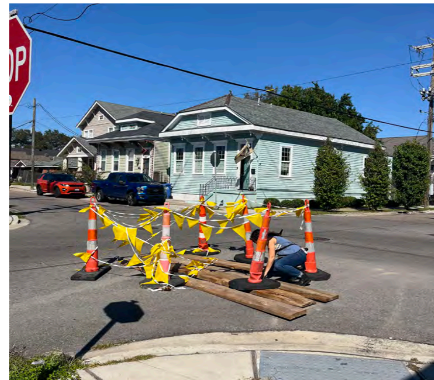
Katie Fisher looking into an active sinkhole, gaged with cones and boards, in New Orleans on November 6, 2025. Photo: Abbie Powers.
